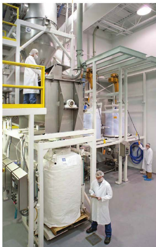
Overall view shows two bulk bag dischargers for whole wheat flour and nonfat dry milk, pneumatic conveying lines, weighing hopper, hand addition of ingredients, the ribbon blender, and final mix in the bulk bag below blender.
